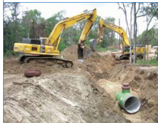
Upper Sabine Basin River Water Supply Project pipeline will augment raw water supplies 50,000 – 80,000 acre-feet per year
