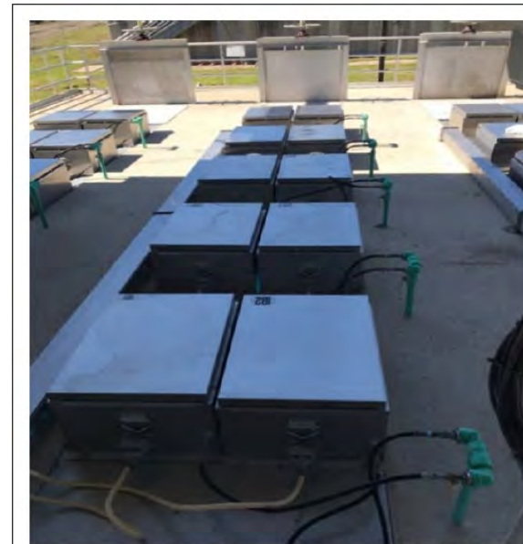
UV 601 – 603 were the first UV units installed at Wilson Creek.
