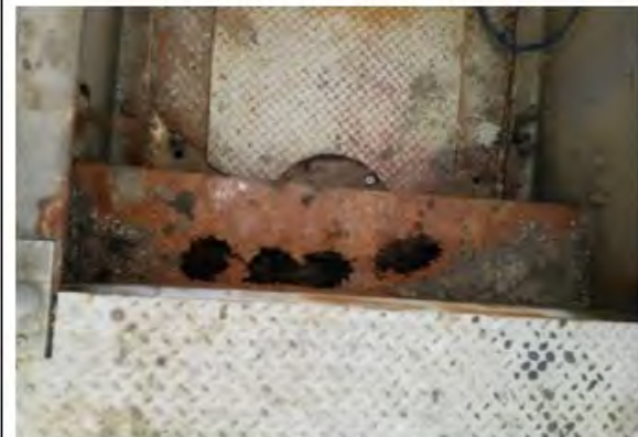
Significant corrosion of stairs atop Plant 1 – South primary tanks
