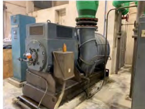
Blower Building 1 has older blowers with limitations in their operation and no HVAC for the building
