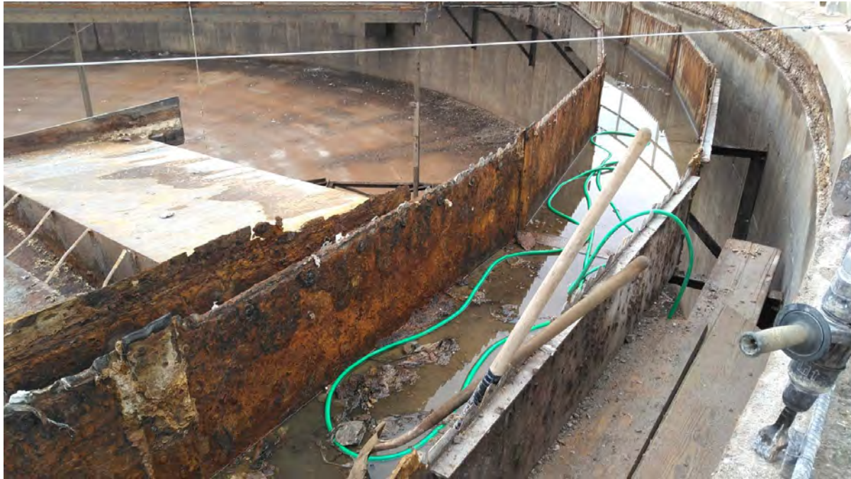
Visible rust, corrosion, and metal delamination
